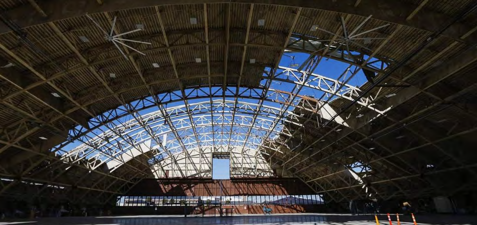
DAMAGED CEILING OF HANGER 5 AT TYNDALL AIR FORCE BASE EARLY IN 2019 – A RESULT OF HURRICANE MICHAEL. TAMPA BAY TIMES PHOTO BY TAILYR IRVINE
